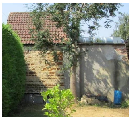
Side view of the workshop showing the original stonework and the point where it was attached to the cottage.
